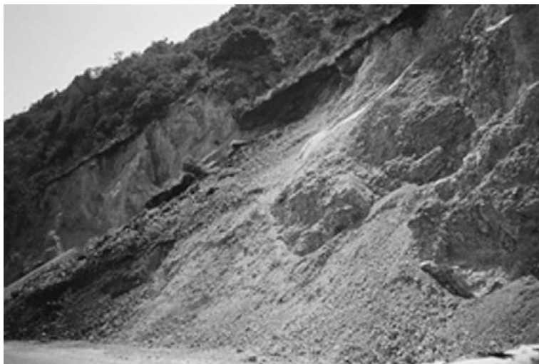
Fig. 7. Landslide on the road Ag. Petros—Kalamitsi (photo taken by Ganas, 25/08/2003).
