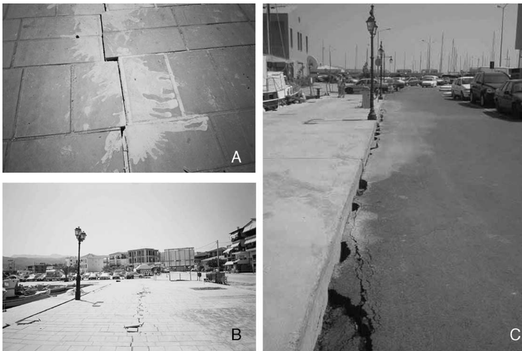
Fig. 10. Liquefaction induced ground failures in the town of Lefkada; (A) sandy silt ejected from ground cracks, (B) ground cracks in the waterfront area, (C) horizontal displacement of the pavement and ejected of sandy material in the marina district (photos taken by Papathanassiou, 15/08/2003).
