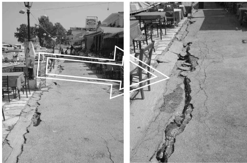
Fig. 14. Ground cracks in the village of Lygia (photo taken by Papathanassiou, 15/08/2003).
