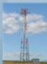
Mobile Base Station Transceiver
