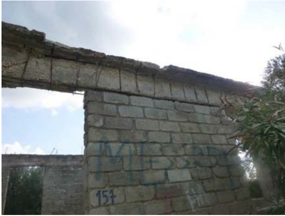
Fig. 9 A wall comprising concrete-block masonry. Note the arrangement of the lintel beam
