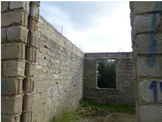
Fig. 10 In the entrance corner of the semi-complete house note the vertical reinforcement as well as the starter bars for lap splicing reinforcement of the second floor at the crest of the first floor perimeter beam
