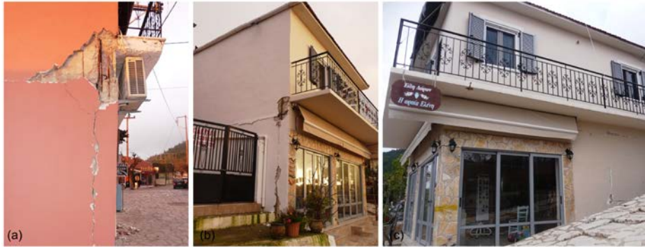
Figure 6. (a-b) Damage to the columns and beam column joints of RC buildings; (c) Large cracks at infill panels in Athani.
