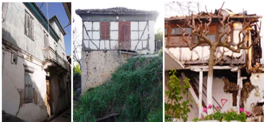
Figure 7. The crack pattern surveyed for the traditional LBSM-TF typology: (a) A previously damaged house in Lefkada town with in-plane diagonal shear cracking; (b) Building in Ag. Petros with wall angle detachment due to soil subsidence; (c) “Red” tagged building in Athani.
