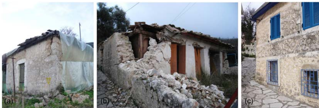
Figure 8. (a) LBSM “yellow” tagged building with separation of walls intersection; (b) characteristic damage of a single floor LBSM-TC; (c) LBSM-RC remained intact after earthquake
